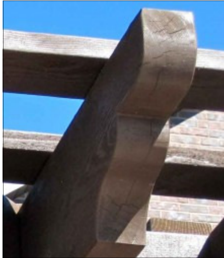
Small “checking” cracks
