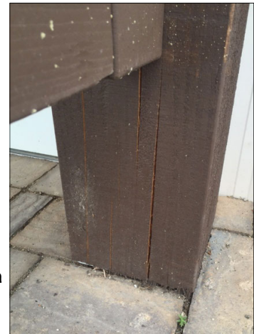
Larger “checking” cracks
