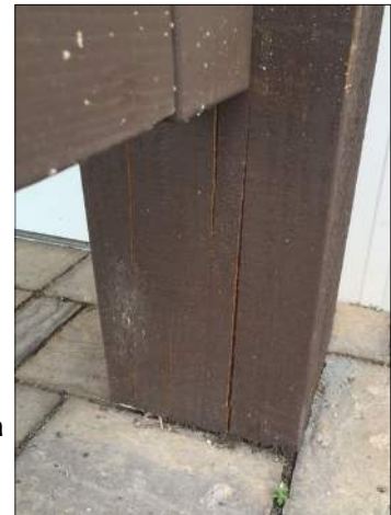
Larger “checking” cracks
