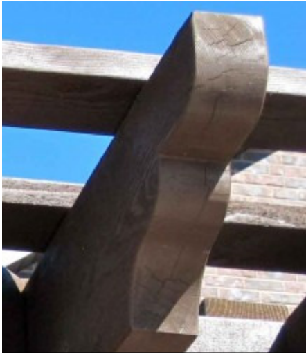
Small “checking” cracks
